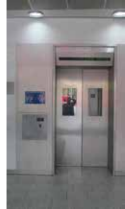
lift doors closed 2.jpg
