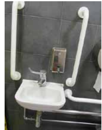
toilet bathroom sink handrails.jpg
