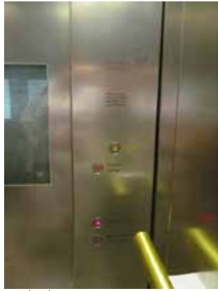
lift inside buttons.jpg
