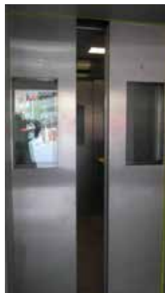
lift doors opening closing.jpg
