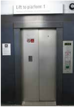
Lift in train station.jpg
