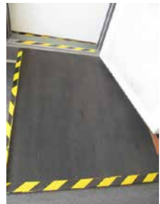
warning tape floor.jpg
